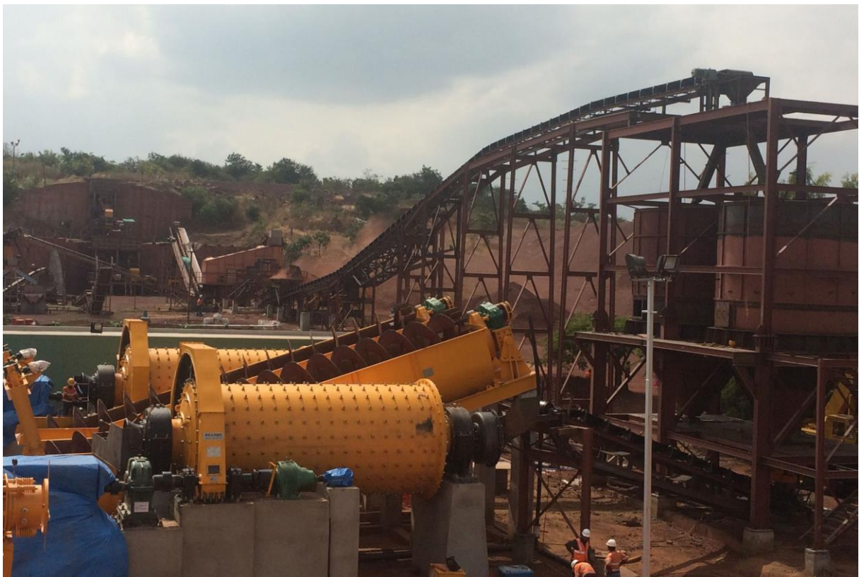
Plant being loaded with first iron ore
