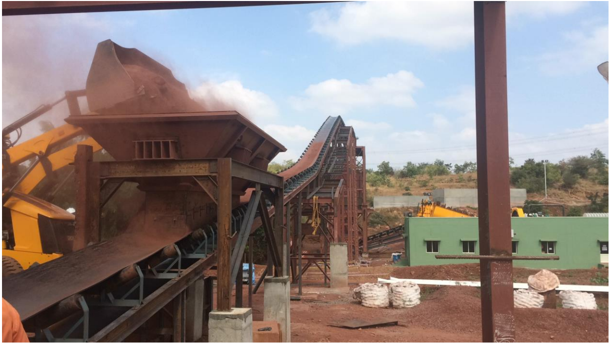
Plant being loaded with first iron ore
