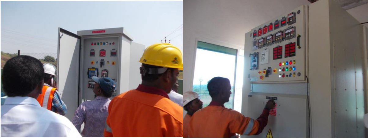
33kV Vacuum Circuit Breaker (VCB) Panel powered up
