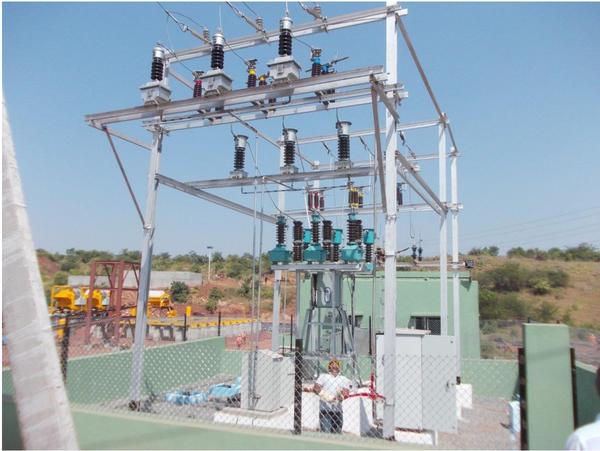
The moment of energisation
