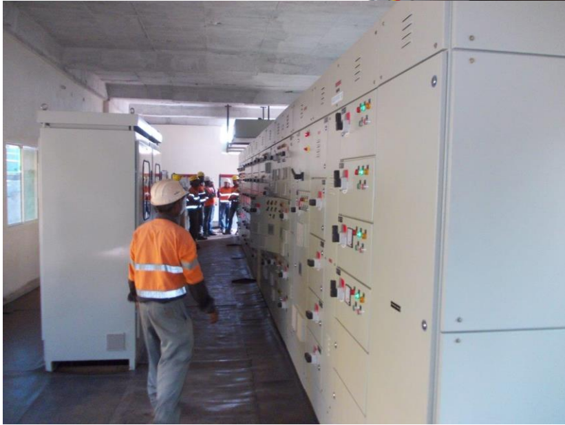
Powered Motor Control Centre (PMCC) Panel powered up
