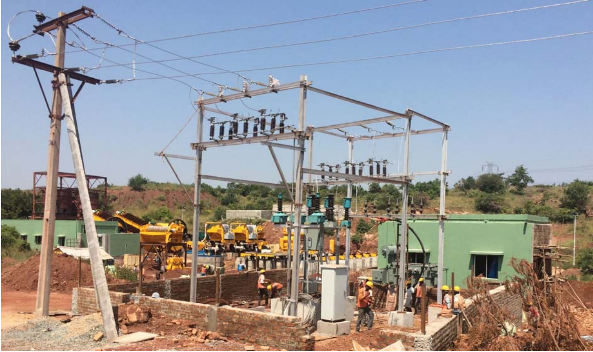
Switchyard to Main Transformer
