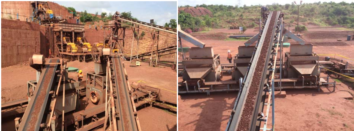
Plant in Operation
